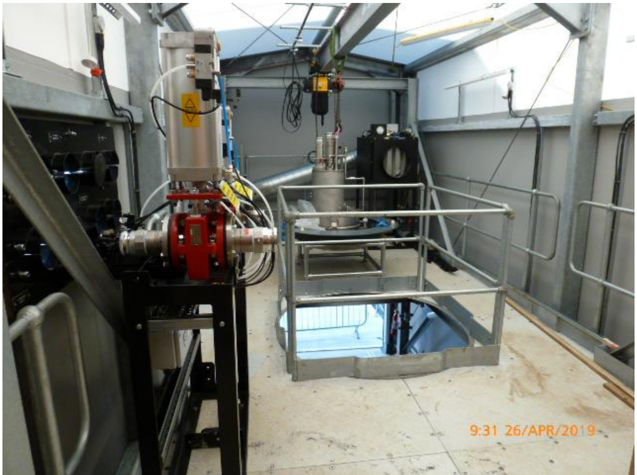
The Fill House building being equipped with retrieval and DCIC filling equipment
