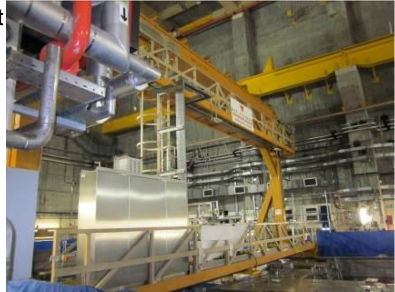
Pond Fuel Handling Machine
